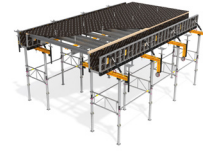
Garage Beam Forming
