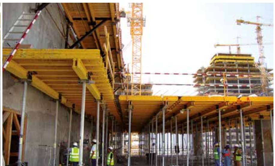
▲ VM-20 beams in Table VR horizontal formwork and for working platforms on climbing brackets
