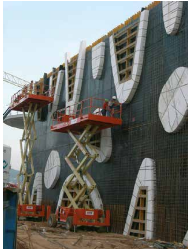
▲ High-quality finish of fair-faced concrete walls with phenolic plywood in ENKOFORM V-100 vertical formwork
